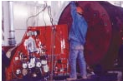
Installation of KBSD steam atomising burner on MISSION™ OL boiler in Qingdao factory.
